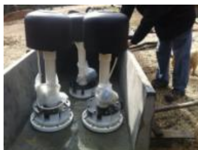
3 x LH turbine concrete flume
