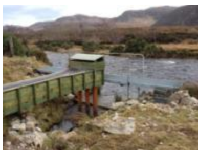
3 x LH turbine timber flume
