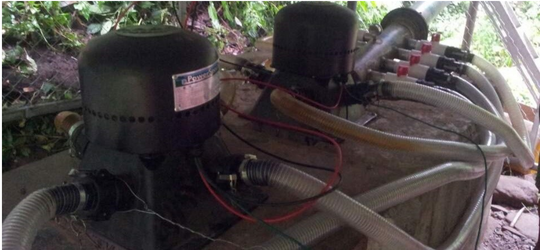
No pipe supports
