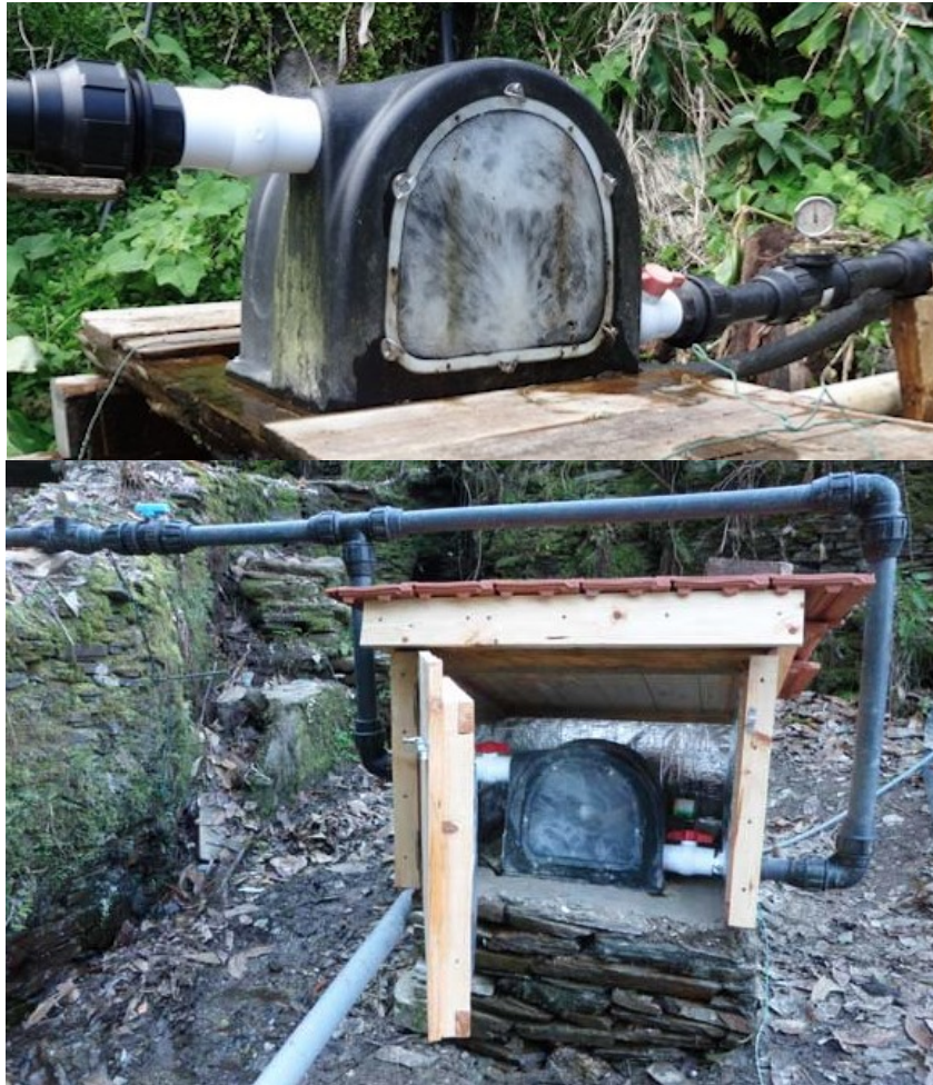
PE pipe and fitting manifolds
