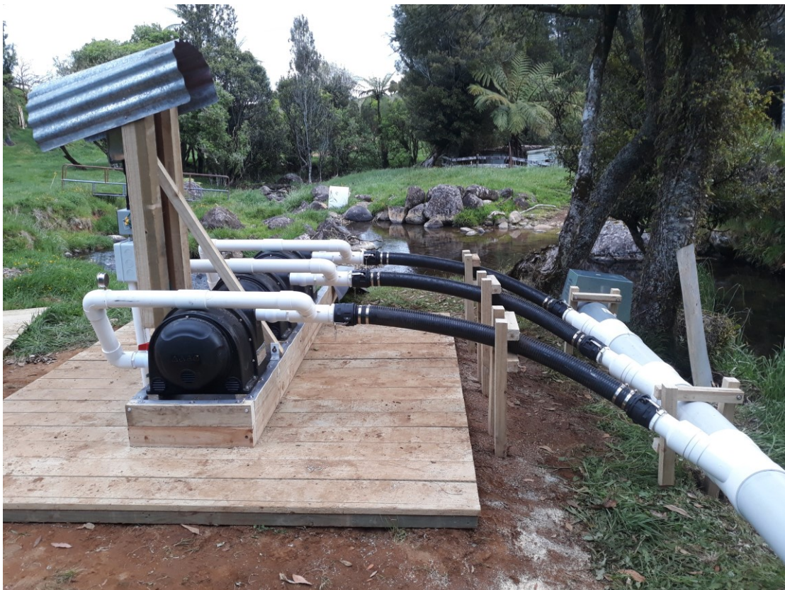
3 x PLT turbines with a combination of PVC and 75mm flexible hoses
