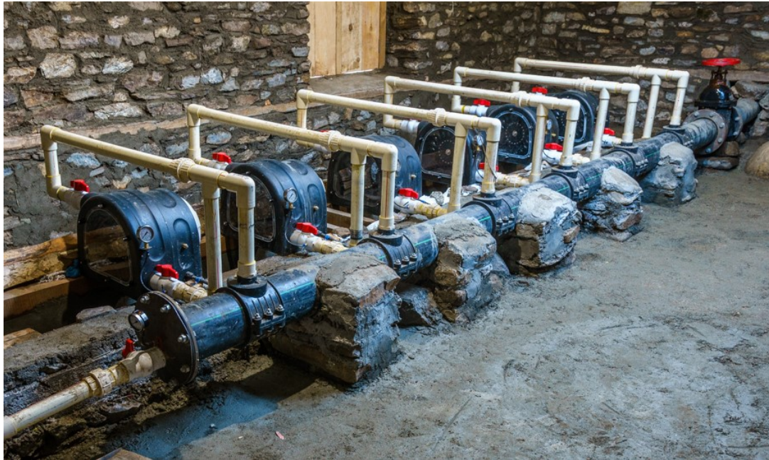
6 x PLT turbines with a combination of PE pipe and PCV manifolds
