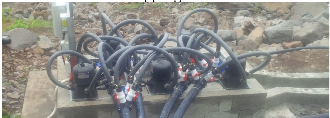
No pipe supports
