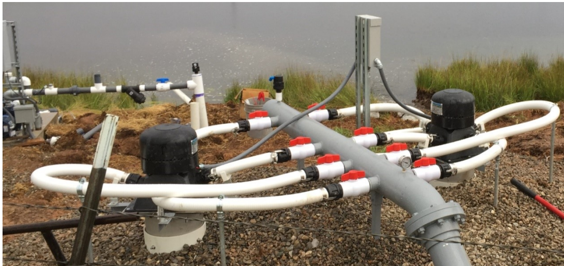
Well installed TRG turbines (steel and flexible pipes)
