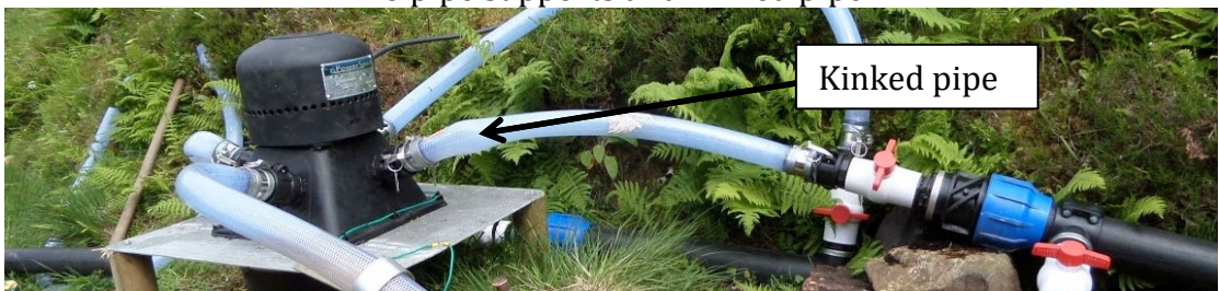
No pipe supports and kinked pipe
