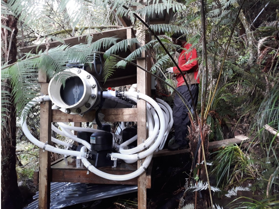
5 x TRG turbines in the process of being installed (steel and flexible pipes)
