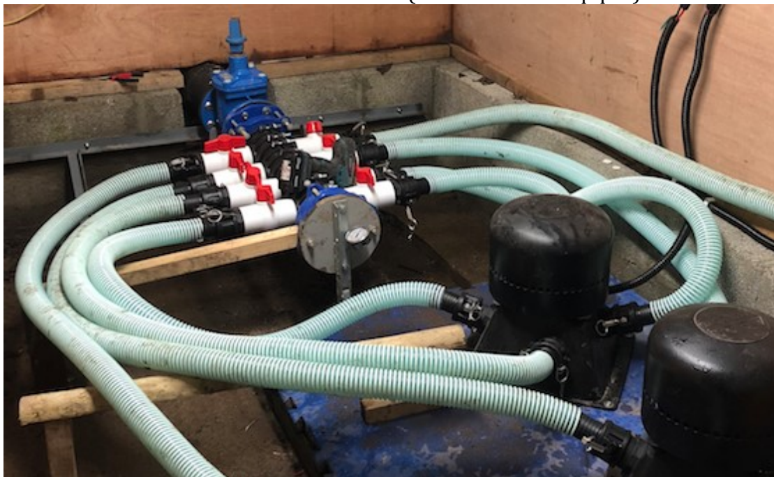
Twin TRG turbines in the process of being installed (steel and flexible pipes) (note jet supports not yet fitted)
