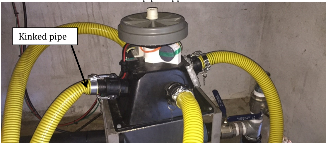
No pipe supports and kinked pipe
